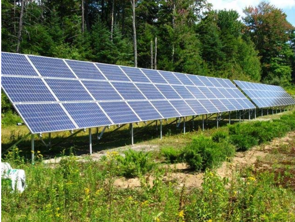
15 KWP PV array, Hermitage Inn, Dover, VT
